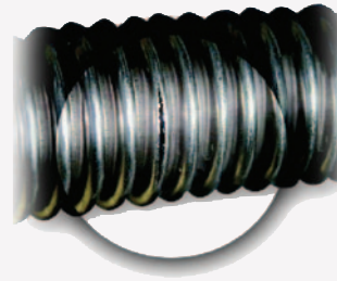
Circumferential cracks on the convolution are typically caused by high velocity flow rates
